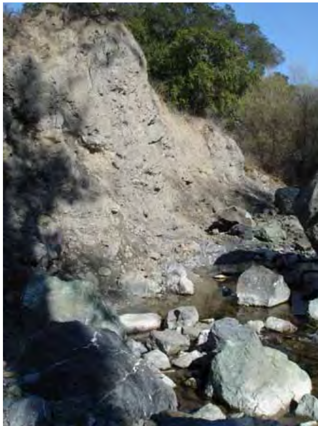
The landslide reach of Arroyo Hondo viewed from downstream on February 3, 2006, (a) with the smaller of two converging landslides visible on the south canyon wall, and (b) the unstable toe of the north landslide where it meets Arroyo Hondo.
